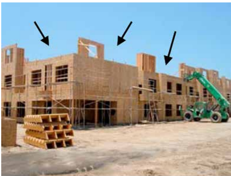
3rd floor work (over 15 feet) requires guardrails. Work here would be in violation of the regulations.
