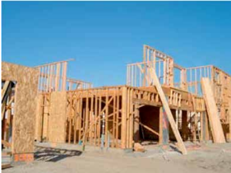
Layout and framing on the 2nd floor (not over 15 feet) do not require guardrails.
